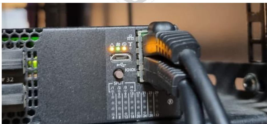
15. Figure: Console and Management Interface of DuT
